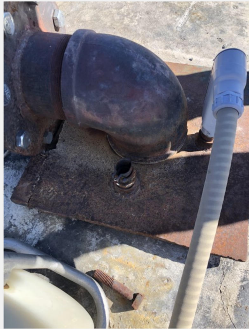
Photograph 6. Access port on steel plate covering well. PVC sounding tube extending into the well casing was not observed.
