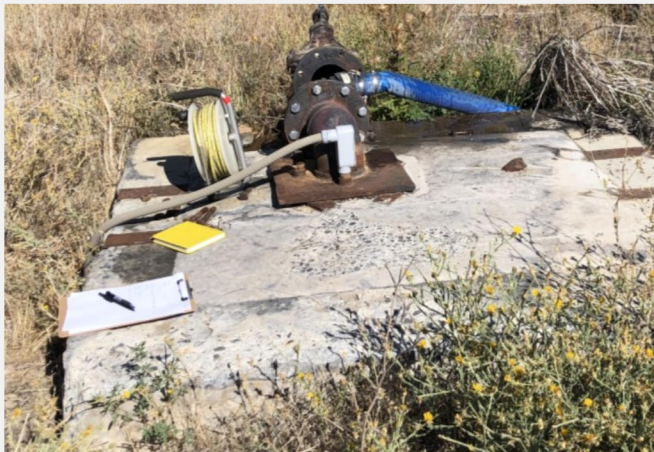
Photograph 7. Gravel feed tube located to the right of the wellhead on the cement pad.
