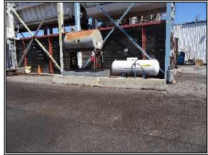
Looking at a 500-gallon gasoline AST and propane tank located to the south of the processing facility.
