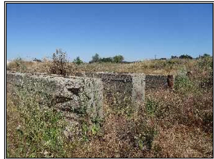
Looking at a second area with concrete foundation remnants on the southwestern portion of the Site.
