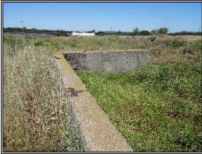
Looking at concrete foundation remnants on the southwestern portion of the Site.
