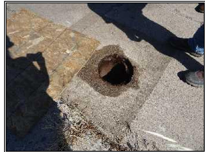
Looking at a 12-inch opening in the concrete pad located on the north-central portion of the Site.
