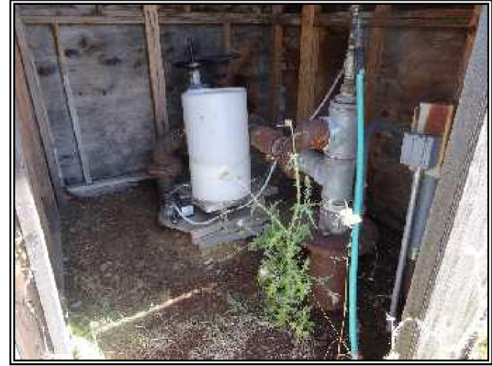
Looking at the well that provides water to the Site.
