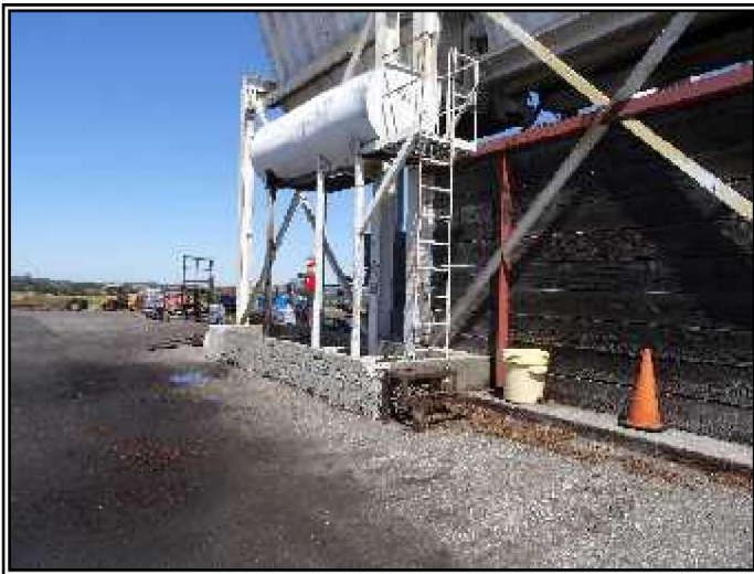
Looking at the 1,000-gallon diesel AST located to the south of the processing facility.
