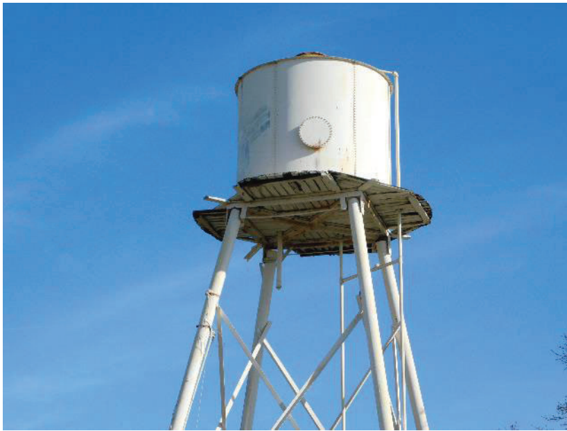
Exhibit 11. Component 11, Water Tank, view to south (Dudek image DSCN8014).
