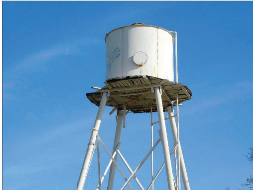
Exhibit 11. Component 11, Water Tank, view to south (Dudek image DSCN8014).
