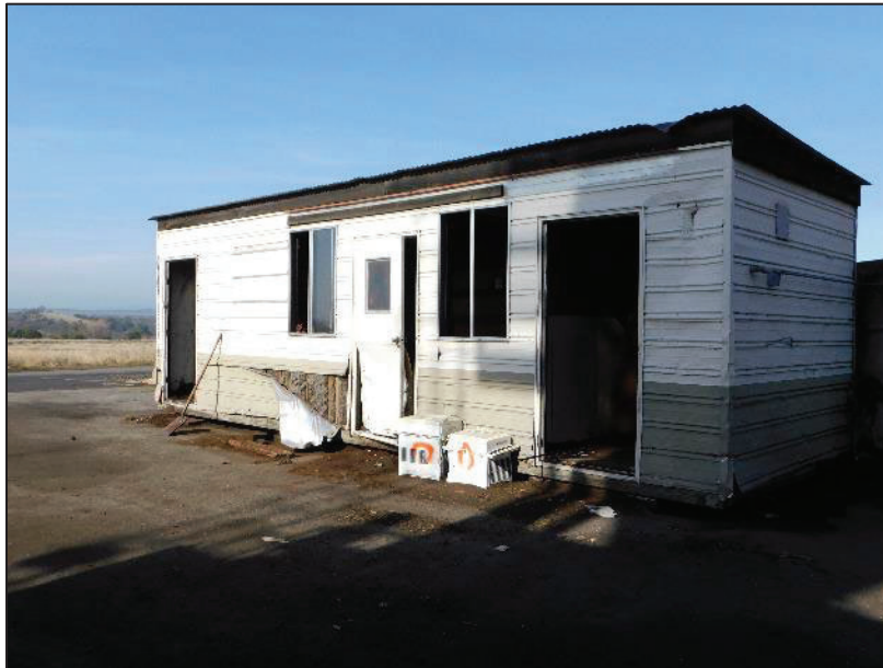
Exhibit 6. Component 6, Office, south and east elevations, view to northwest (Dudek image DSCN7932).
