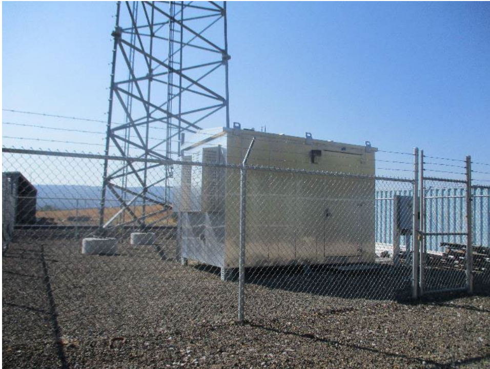
Photograph 26. Mechanical Infrastructure, view looking northwest (IMG_526).
