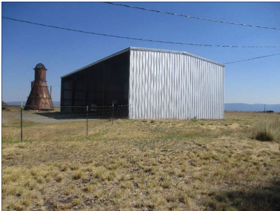
Photograph 8. Storage Barn C, west elevation and open north side, view looking southeast (IMG_458).
