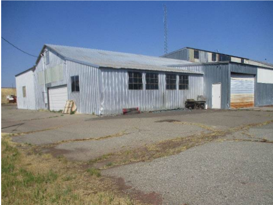
Exhibit 6. Map ID. 1C, Warehouse, west and south elevations, showing multiple additions. View looking northeast (IMG_508).
