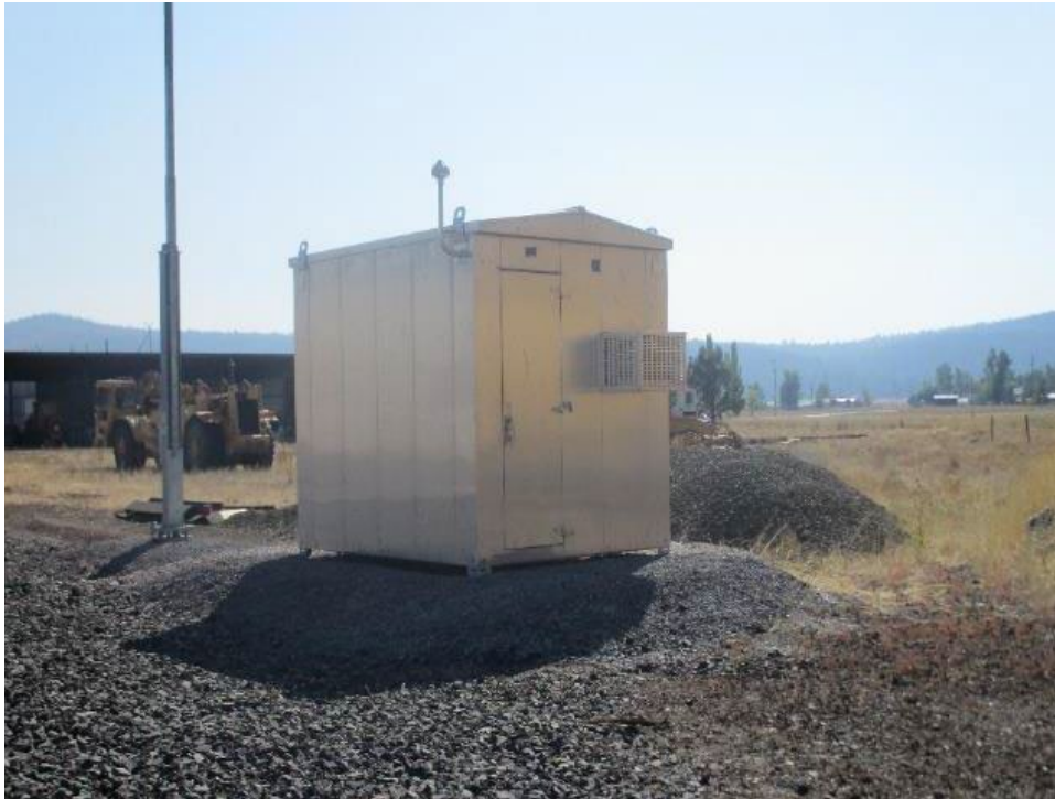
Exhibit 28. Map ID. 2N, Electrical Shed, view looking southwest (IMG_521).
