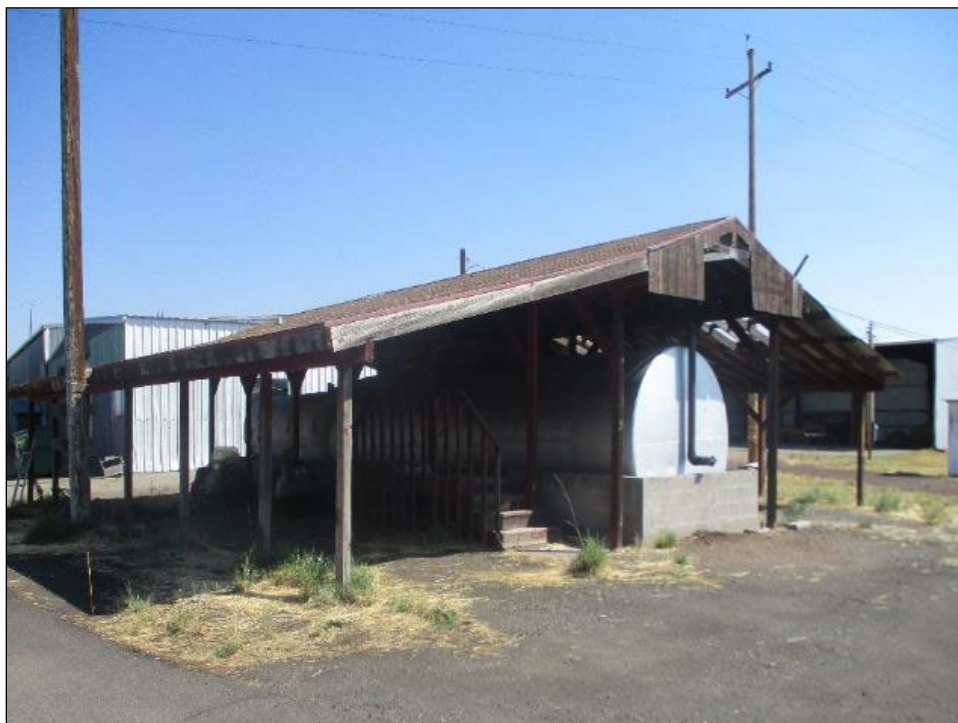
Photograph 10. Propane Shelter, view looking southeast (IMG_469).
