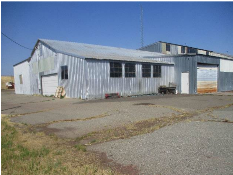
Photograph 6. The Warehouse, west and south elevations, showing multiple additions. View looking northeast (IMG_508).
