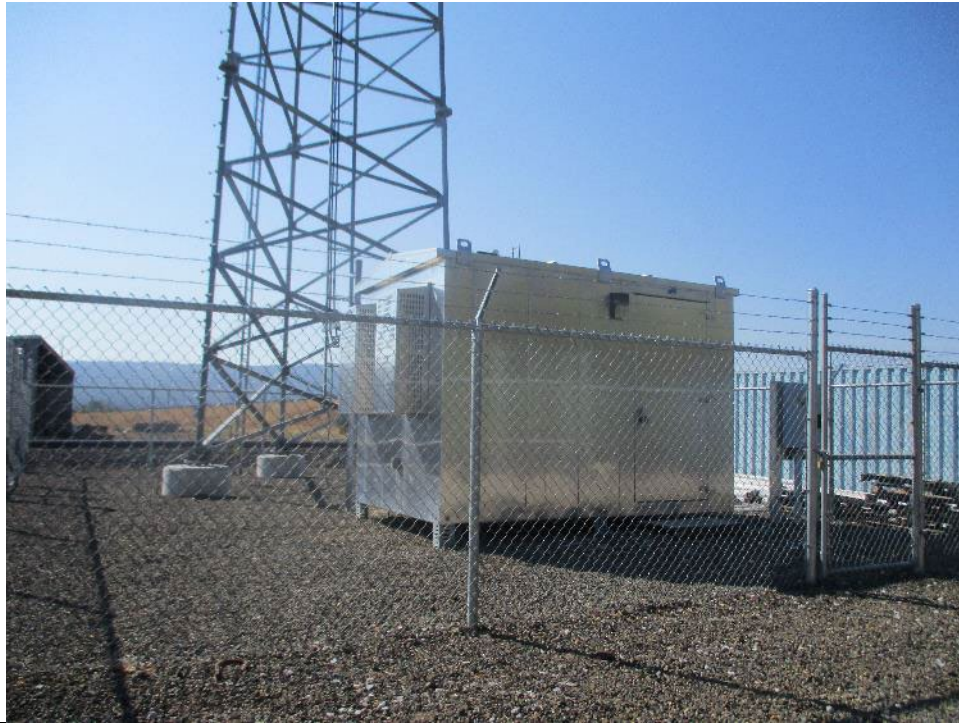
Exhibit 26. Map ID. 2H, Mechanical Infrastructure, view looking northwest (IMG_526).
